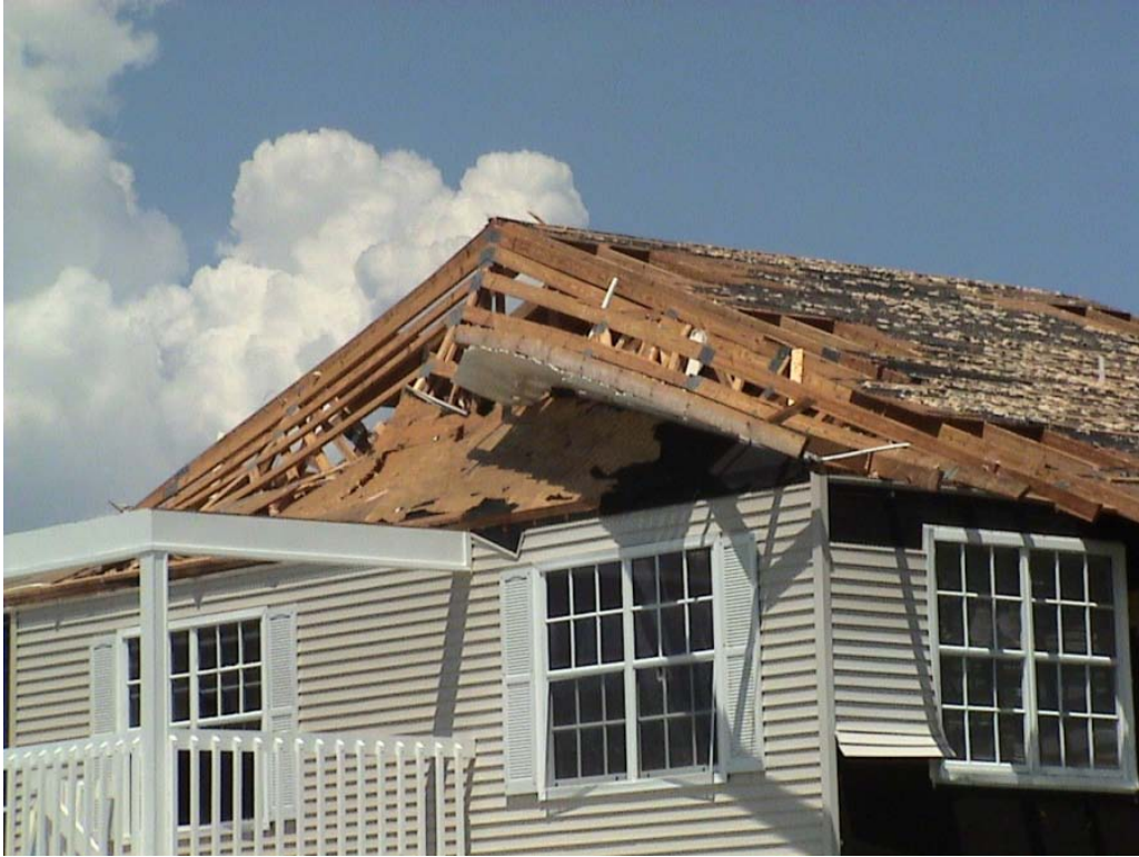
Figure 1.7 The most common gable end failure is one where the wall loses support along its top edge because sheathing is blown off at the overhang. The wall may fold outward (see cover picture) or be blown inward.
