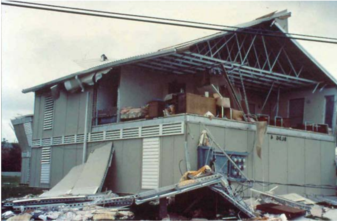
Figure 1.9 The more usual result of wall connection failures is a completely detached gable end wall and the wall below. This building is in the same project as that shown in Figure 1.8. These occupants were not so lucky. Probably all the possessions in this view were saturated with rain water.
