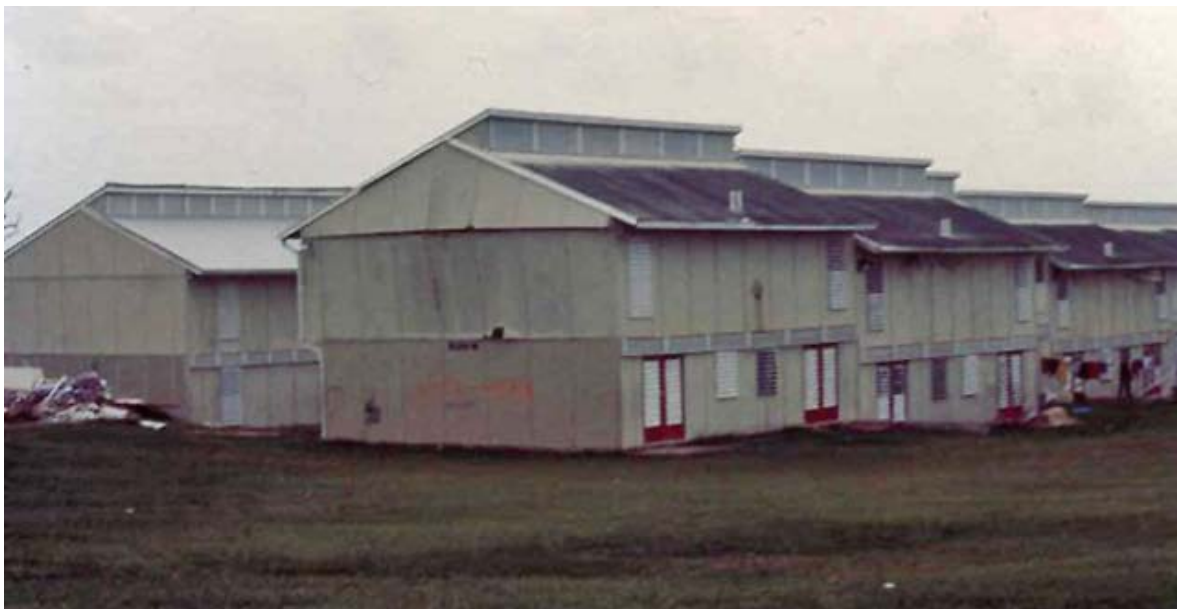
Figure 1.8 The second most common type of gable end failure is at the connection between the rectangular and triangular walls – Here the failure is just at the precipice of coming off the wall. It is the negative pressure of the hurricane that pulled on the gable end wall to compromise this connection when wind blew on other faces of the house to create that negative pressure.
