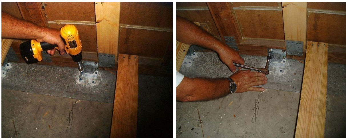
Figure 10.2. This shows an HGAM being installed directly to the top of the masonry wall. Here the elevation of the bottom chord was just fine as well as the grout in the concrete block being fine too.
