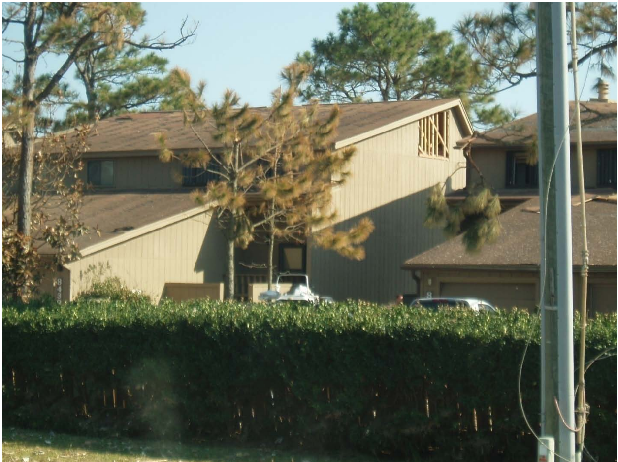
Figure 13.1. Missing siding pulled off by negative pressure or by wind that got into the house and pressurized it causing the siding to pop off. . If the wind shifted direction to blow rain into that opening, the damage to the rooms nearby could have been dramatic. Note plywood (or whatever) on the lower roof on the right.
