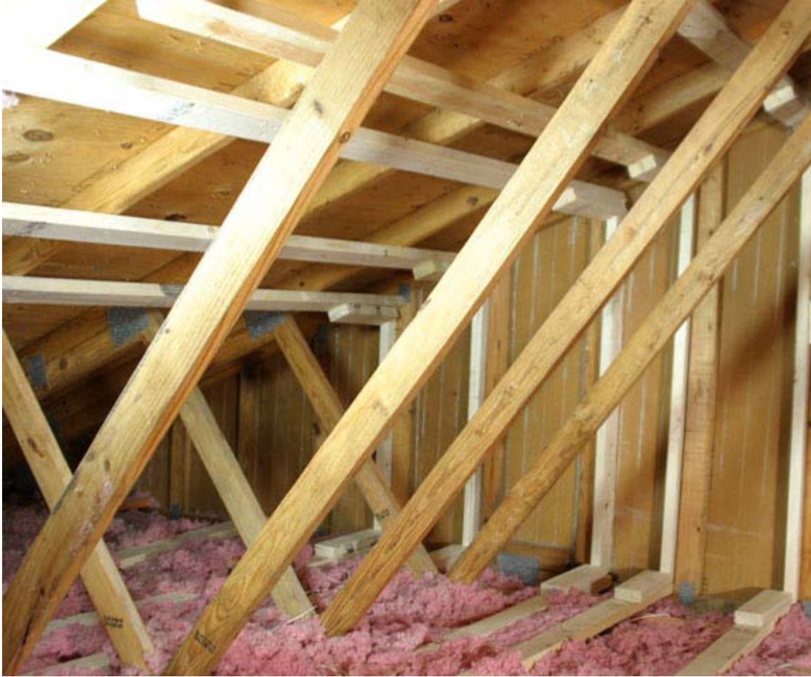
Figure 2.2 Photograph of completed gable end retrofit using the L-bent strap method – the light colored wood is the lumber added during the retrofit activity
