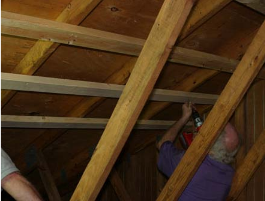
Figure 8.1. Installation of upper horizontal brace by having started screws before lifting the brace up to fasten it.
