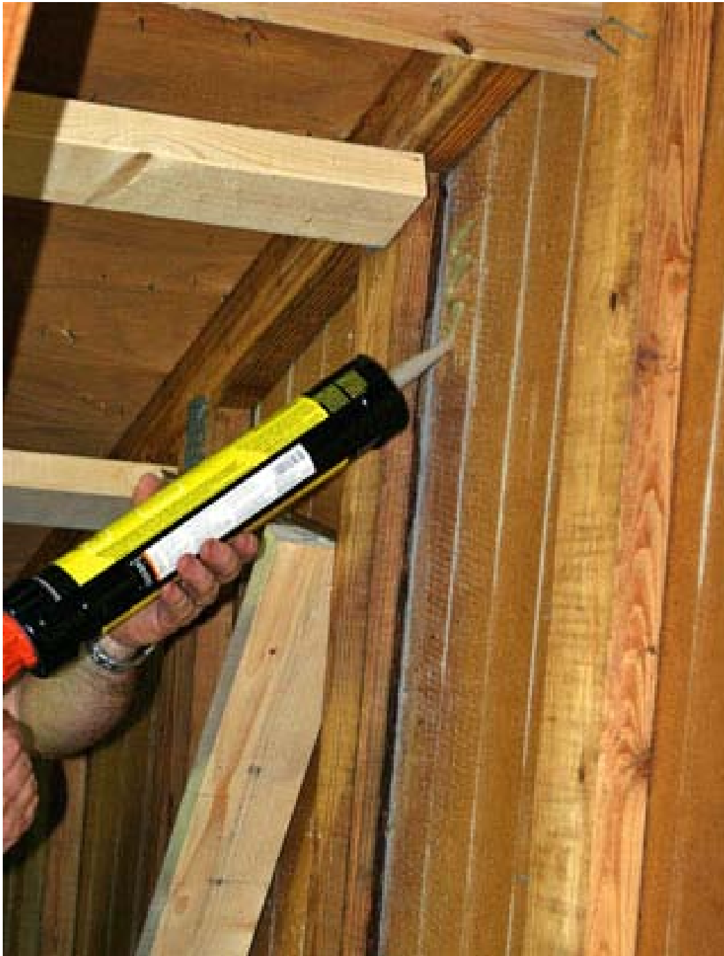
Figure 8.2 Applying construction adhesive where retrofit stud will make contact with the sheathing because it was assumed the sheathing was not sufficiently nailed. An L-strapped retrofit stud is shown about ready to be installed.
