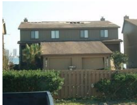
Missing panels from the middle of roof indicates poor nailing of sheathing (click image for larger version)
