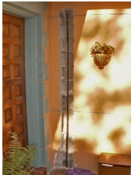
Masonry block cut out to allow steel reinforcing to be added - short pieces are epoxy grouted into the foundation and into the bond beam at the top of the wall.
