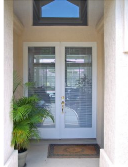
French doors frequently burst open during strong hurricanes.
