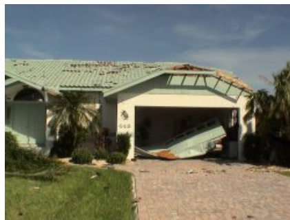
Garage door blown in on top of car. Note the loss of roof sheathing over the garage.
