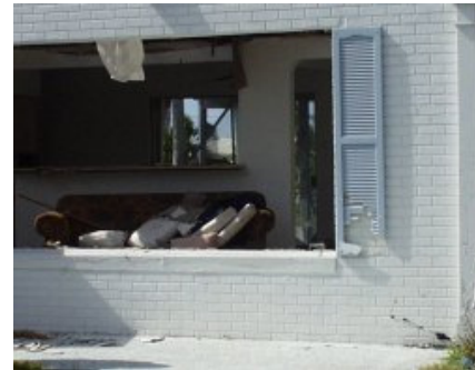
This window and frame was pushed in by the wind.
