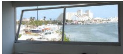
Poorly attached frames can break loose in high winds - this one was pushed out to relieve internal pressures.
