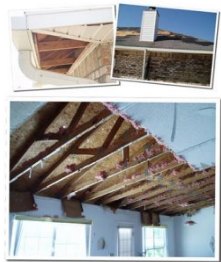
Some roof cover damage plus some soffit damage equals significant interior water damage
