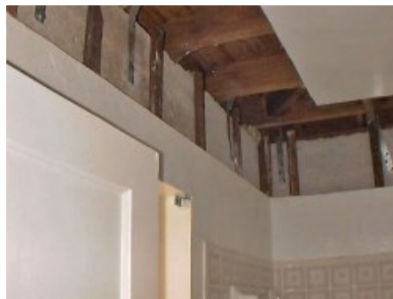
Example of a roof-to-wall connection on a masonry home performed from the inside of the house.
