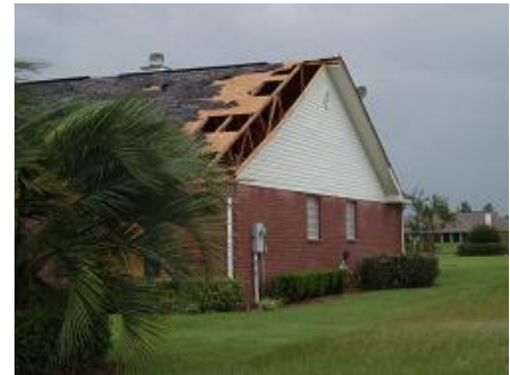
Roof sheathing loss at gable end. This is a common failure point.
