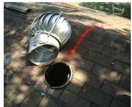
Turbine vent and the hole in the roof
