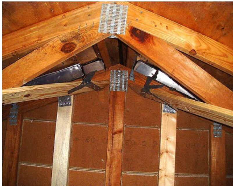
Note aluminum flashing installed and caulked to block water entry during hurricane (click image for larger version)
