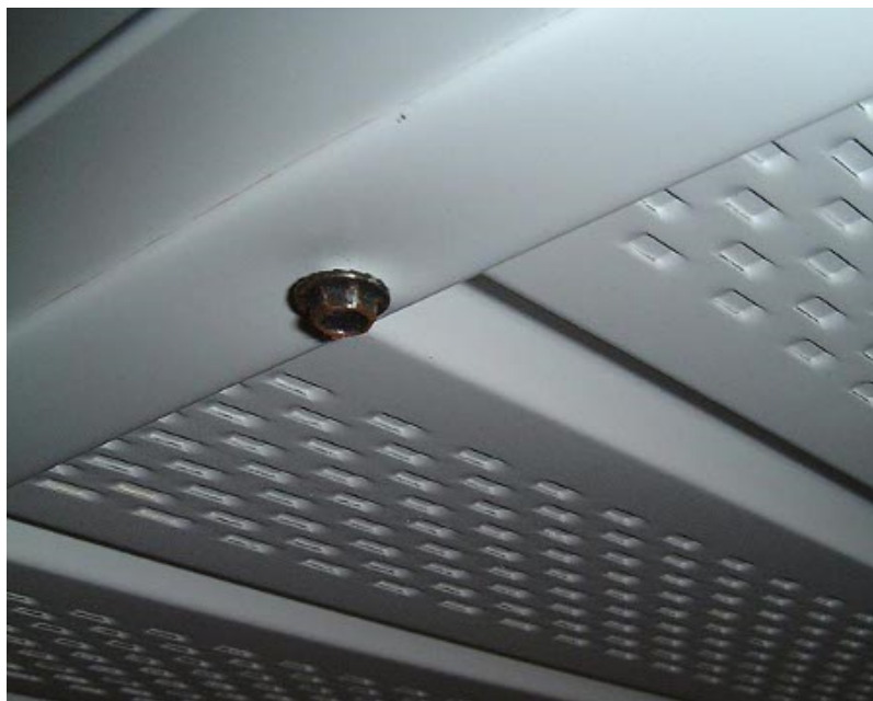
Screw inserted through edge of fascia cover, through soffit panels and into fascia board (click image for larger version)
