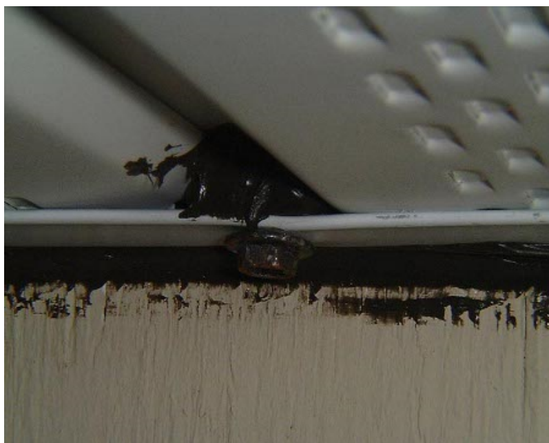
Screw installed through wall J channel and through soffit panel and hopefully into wood above – black caulk shown for contrast. You can usually find screws that also match trim color. (click image for larger version)
