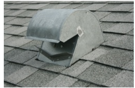
This shows a gooseneck that has had a field applied deflector added to it
