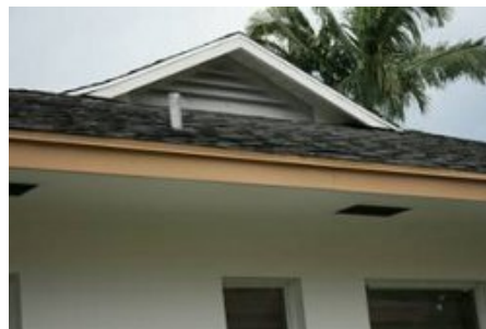
Triangular gable end vent on a Dutch hip gable end. Note soffit vents on the eave.
