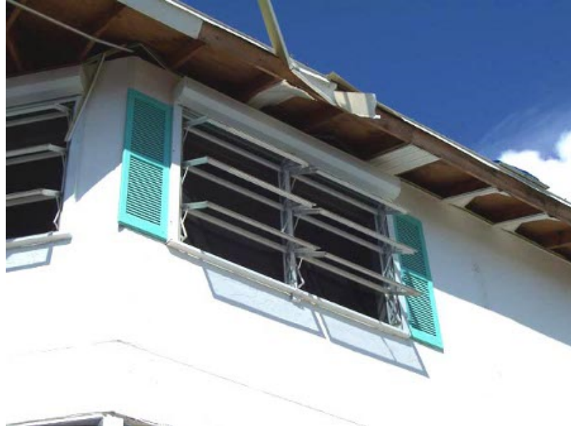
Soffit damage was widespread – this photo shows both fascia cover and wall track damage
